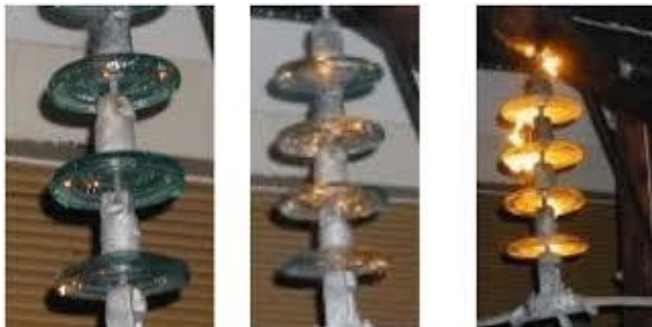
Fig.1.9 Process flashover on polluted insulator
