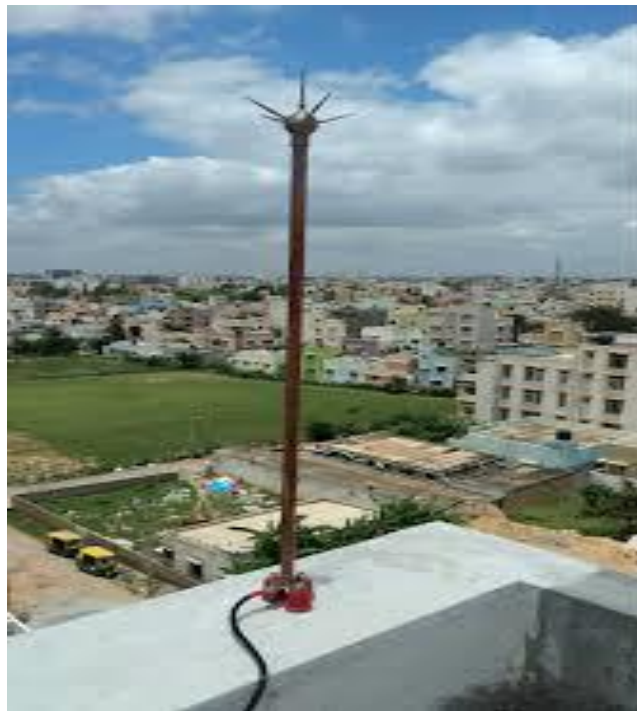
Fig.1.7 Lightning arrester for building
