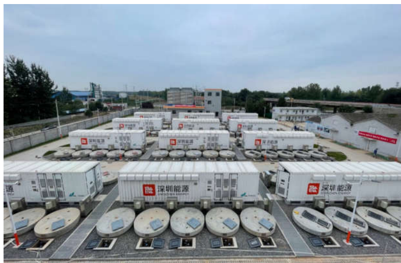
Fig 4. A project in China, claimed as the largest flywheel energy storage system in the world, has been connected to the grid.
